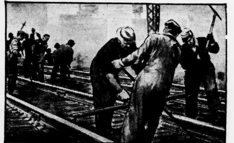
AUGUST... Miles of track relaid—re-ballasted—almost 29,000 tons of rail installed for the year—in spite of shortages of men and materials. It is only by constant inspection and careful maintenance, that our right-of-way is able to stand up under the strain and stress of wartime traffic.
