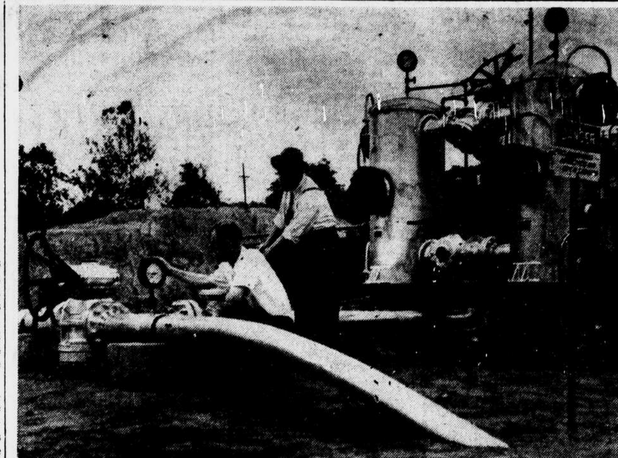
THE DISTRICT'S FIRST PIPELINE—Shown above is the local terminal of the new 6-inch pipeline of the Sinclair Refining Co., which will bring gasoline, fuel oil and other petroleum products directly into the District. H. H. Magee, Sinclair company inspector (left), is looking at the pressure gauge, which shows a pressure of 900 pounds a square inch when the line is delivering its full capacity of 21,000 gallons an hour. A. N. Harris, construction engineer, is operating the valve.—Star Staff Photo.
