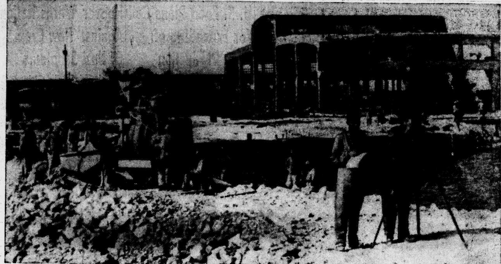
TRIPOLI.—RECONSTRUCTION WORK—View of the famous mole at this Libyan harbor, heavily battered by the Allies while the port was Axis-held. It is now being rebuilt under Allied direction. Note surveyors at right. —A. P. Wirephoto.
