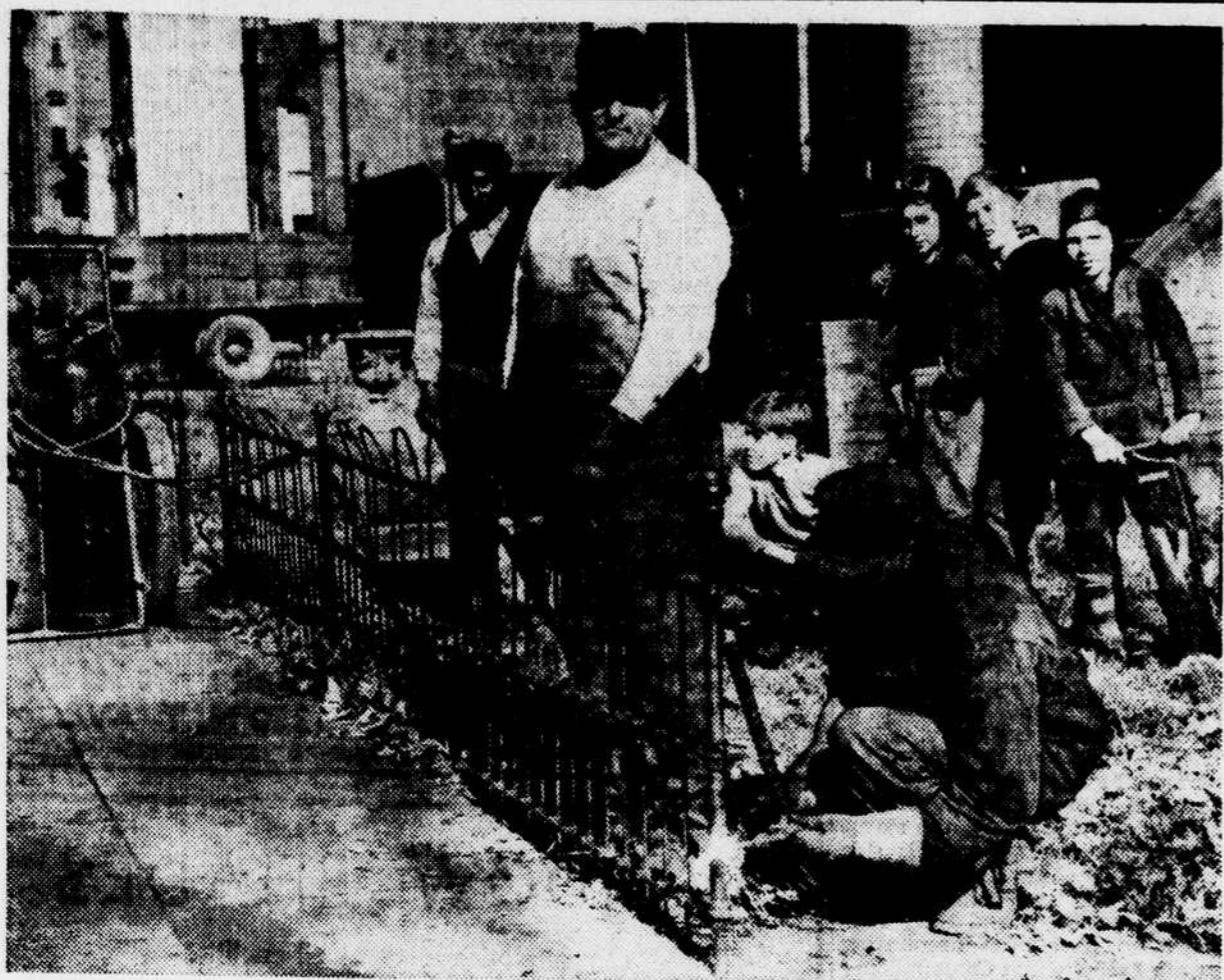
FENCE FOR VICTORY —As the campaign to salvage District fences, railings and ornamental grill-work gains momentum, William Smith, local scrap iron dealer, supervises the work of one of his laborers, Alf Johnson, who applies an acetylene torch to property owned by Mr. Smith's father, Joseph Smith, at 719 Mount Vernon place N.W. This fence measured approximately 112 lineal feet, weighed approximately 1,000 pounds. —Star Staff Photo.
