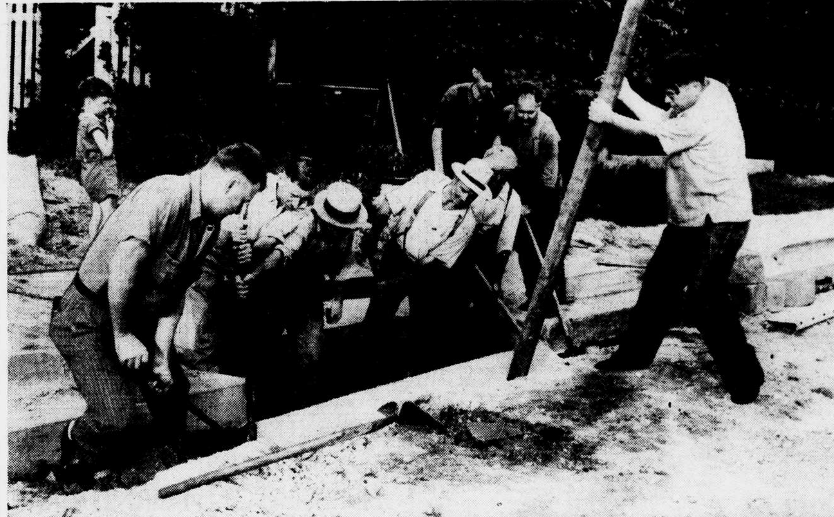
SEAT PLEASANT OFFICIALS REPAIR OWN STREETS—Labor shortage hasn't stopped improvements on Seat Pleasant streets. Here members of the council are shown helping in street repair. Left to right are Van Moreland, Mayor; Joseph Wells, council-
