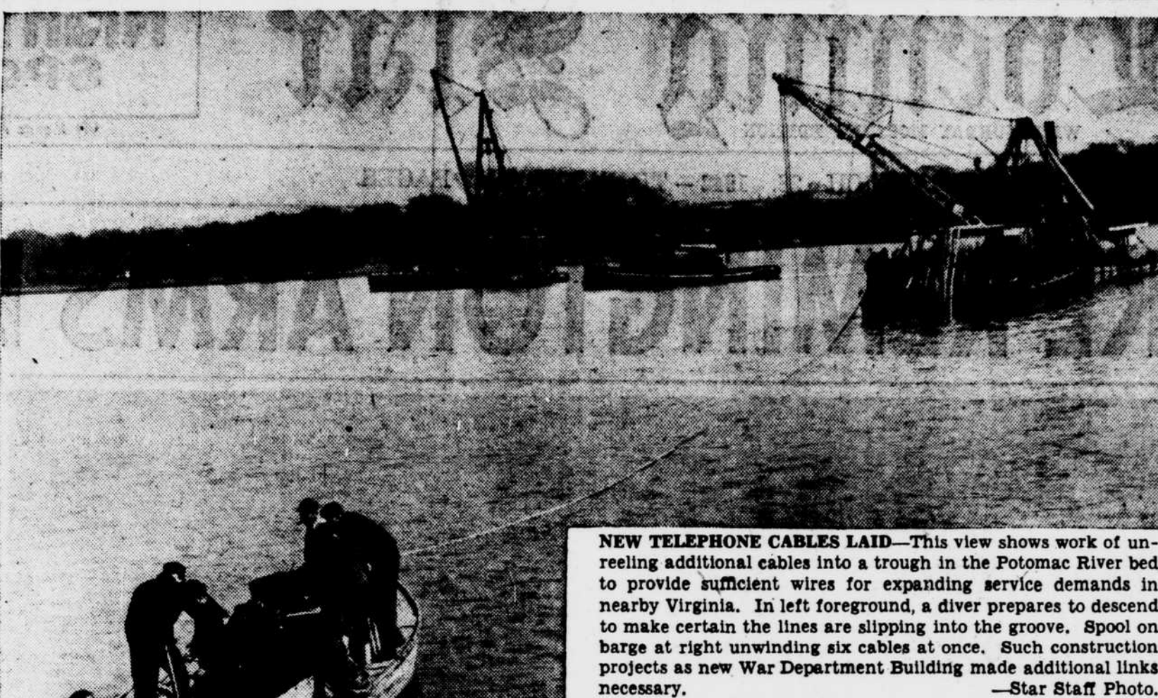
NEW TELEPHONE CABLES LAID—This view shows work of un-reeling additional cables into a trench in the Potomac River bed to provide sufficient wires for expanding service demands in nearby Virginia. In left foreground, a diver prepares to descend to make certain the lines are slipping into the groove. Spool on barge at right unwinding six cables at once. Such construction projects as new War Department Building made additional links necessary. —Star Staff Photo.
