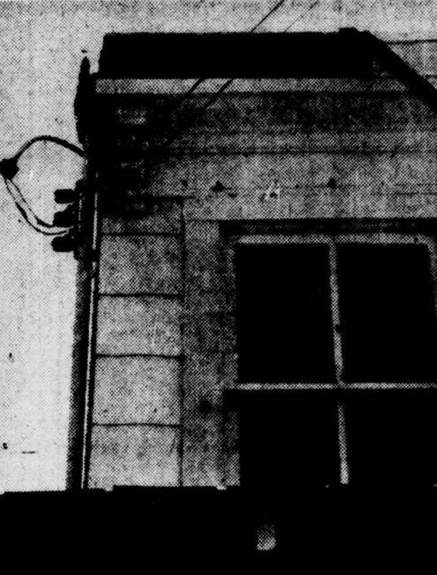
The roof of the home of Miss Clara Derry of 101 Sixty-first street, Capitol Heights, first was damaged by a flying section of the broken wheel, which ricocheted off.
