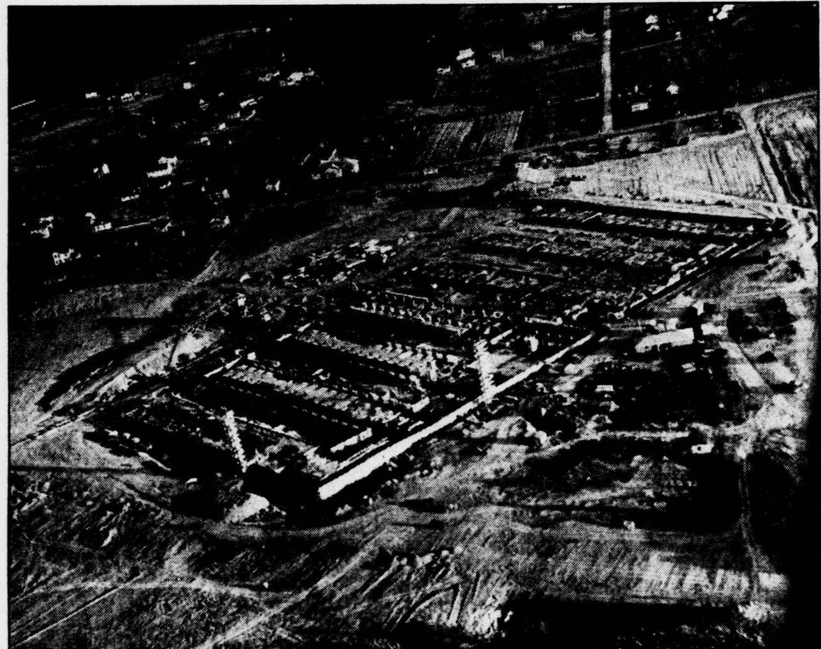
FEDERAL OFFICE BUILDING RISING AT SUITLAND, MD.—This air view of Federal Office Building No. 3 at Suitland, Md., looking southeast, shows progress of construction on the $4,100,000 project scheduled for completion next spring. The Silver Hill road crosses the picture beyond the 430-acre building site and the Suitland School can be seen in the center background facing the road. The Suitland road intersects from the left. The building will house about 4,500 workers and is about 6 miles from the Capitol. The Washington Suburban Sanitary Commission is selling a bond issue to provide funds for water and sewer facilities and special zoning powers have been granted Prince Georges County commissioners to protect the area. It has not been decided what offices will occupy the building. —Photo by Bill Young.
