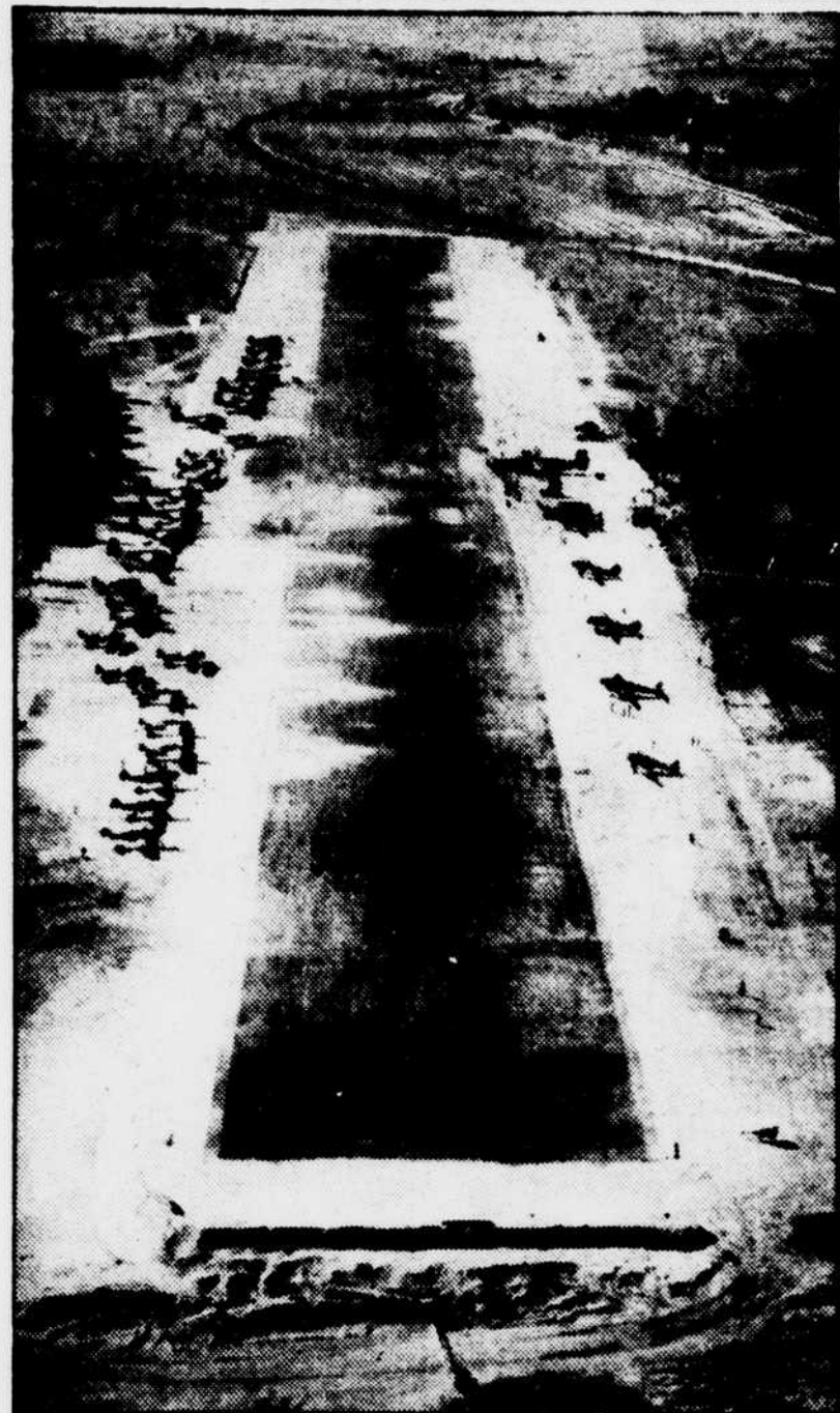
MARSTON, N. C.—TEN DAYS TO BUILD AIR FIELD—A portable landing strip set up by Army engineers in 10 days near here is being used by the Air Force attached to the 1st Army Blues for its war maneuvers battle against the 4th Corps. The landing strip is made up of metal grating in strips 10 feet long and 18 inches wide, transported by truck and fastened together upon arrival at the desired spot. —A. P. Photo.
