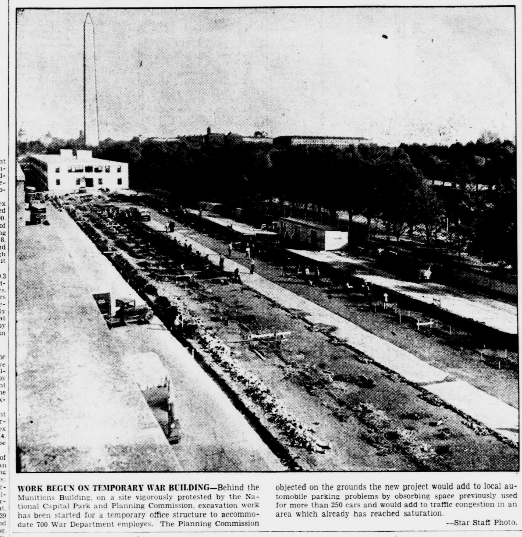
WORK BEGUN ON TEMPORARY WAR BUILDING—Behind the Munitions Building, on a site vigorously protested by the National Capital Park and Planning Commission, excavation work has been started for a temporary office structure to accommodate 700 War Department employees. The Planning Commission objected on the grounds the new project would add to local automobile parking problems...
