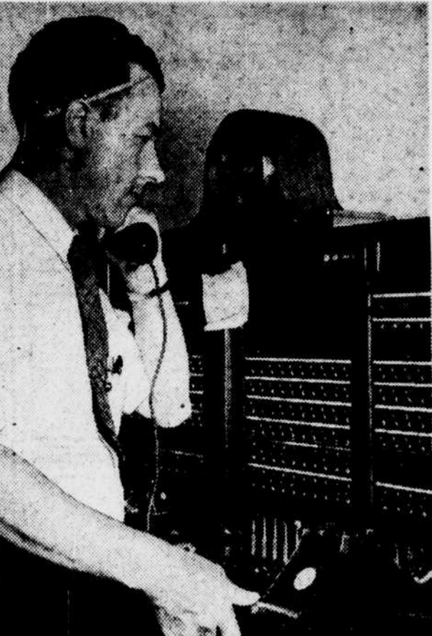
Thomas Phillips, a fire alarm operator, works the special switchboard at fire alarm headquarters, set up for the tests with color signals marking progress of the raid.
