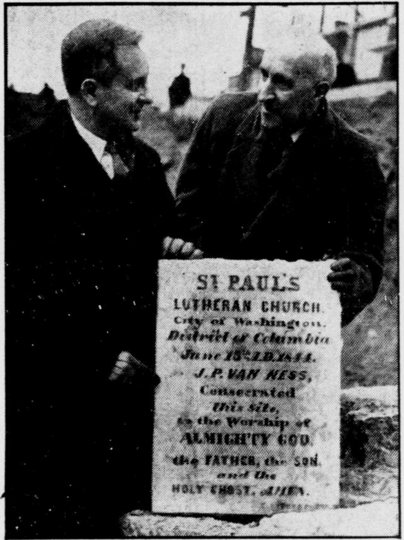
TURNED UP IN A SHOVEL—This cornerstone of old St. Paul's English Lutheran Church, laid in 1844, was unearthed yesterday by a steam shovel excavating at Eleventh and H streets N.W. for construction of an office building. The cornerstone, left 10 feet underground when the site was filled in for a parking lot about 10 years ago, contained a Bible, papers and eight coins. Shown examining the tablet which covered the stone crypt are Dr. Henry W. Snyder (left), pastor of the new church at Connecticut avenue and Everett street N.W., and Luther W. Linkins, chairman of the church Building Committee.—Star Staff Photo.
