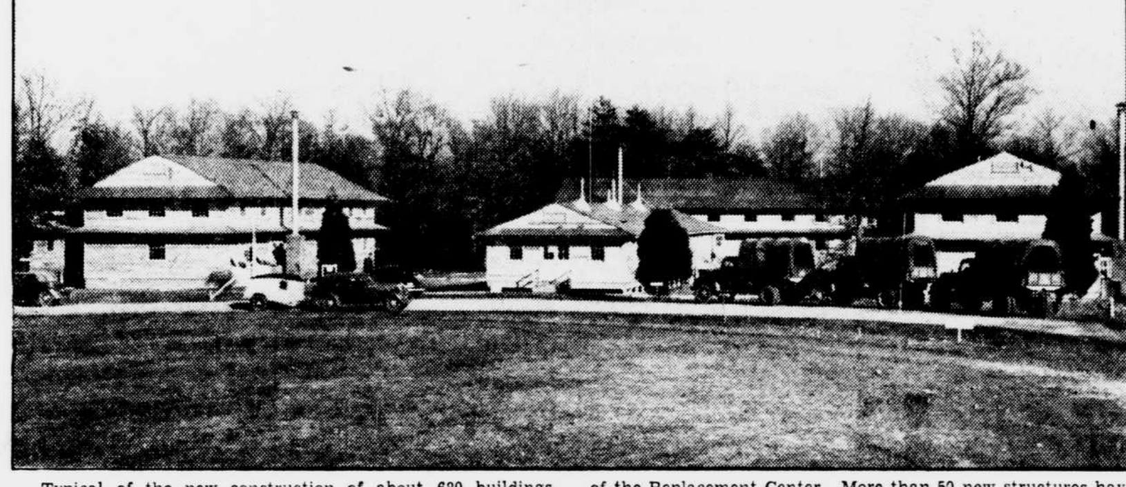
Typical of the new construction of about 680 buildings being erected by the Charles H. Tompkins Co. of this city to house the spring flood of selectees in this group of two-story barracks and one-story mess hall, now used as headquarters
